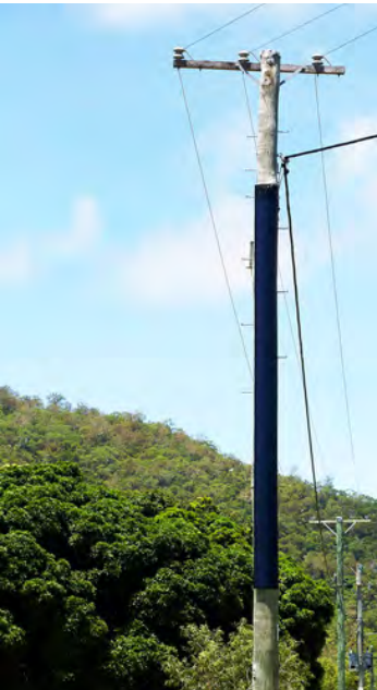
Figure 186 Example of curved PV panel installed on utility poles directly may be a more attractive alternative
