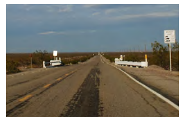
Figure 164 Timber trestle bridge east of Danby Rest Area that still retains historic wood parapet rail with metal 'W'-beam approach rail attached
